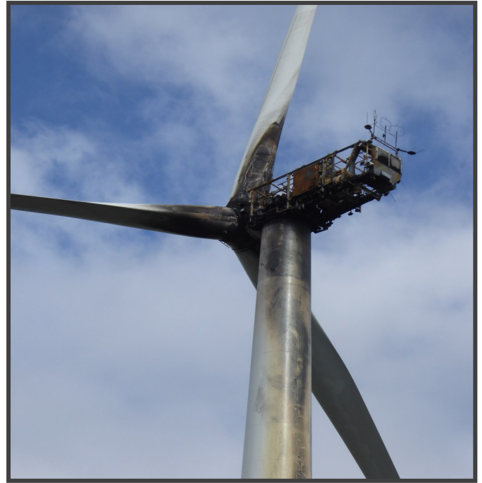
Wind Turbine Failure, U.K.
